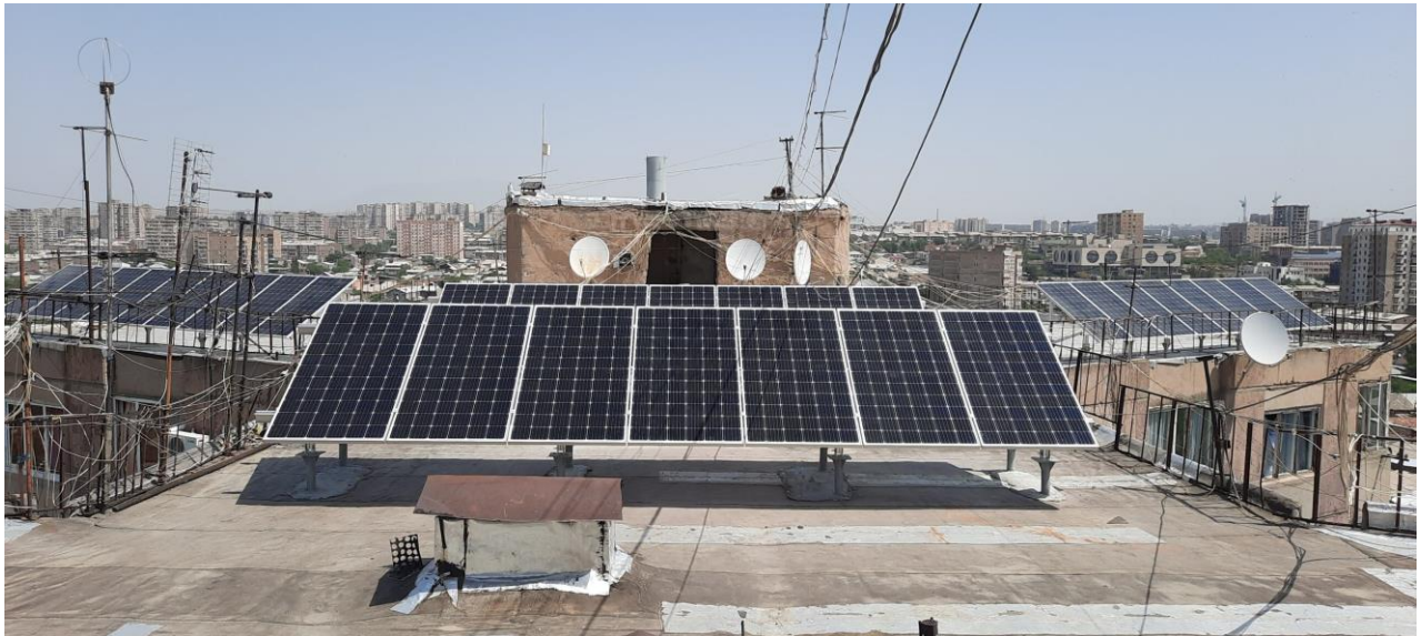
Fig. 1. EU4Yerevan-Solar Community Project. Solar PV system installed on the roof of multi-story residential apartment building. https://com-dep.eu/eu4yerevan-solar-community-project-promotes-renewable-energy-energy-efficiency-retrofits-in-multi-apartment-buildings/
